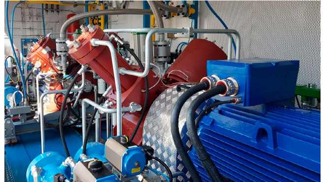
Installation of compressors in tandem with control systems
